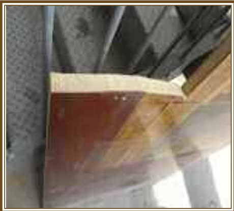
The "thickness" of the damage
